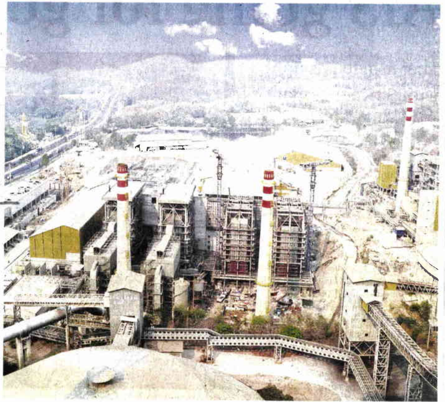
TPIPP's power plant in Saraburi, with capacity of 220 megawatts, has begun operations.
