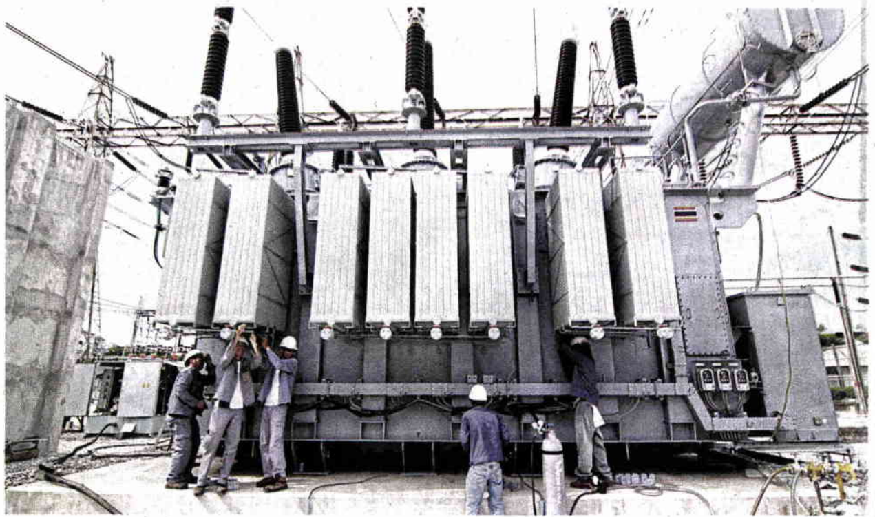
TRT makes and installs transformers for business operators and state power utilities.
