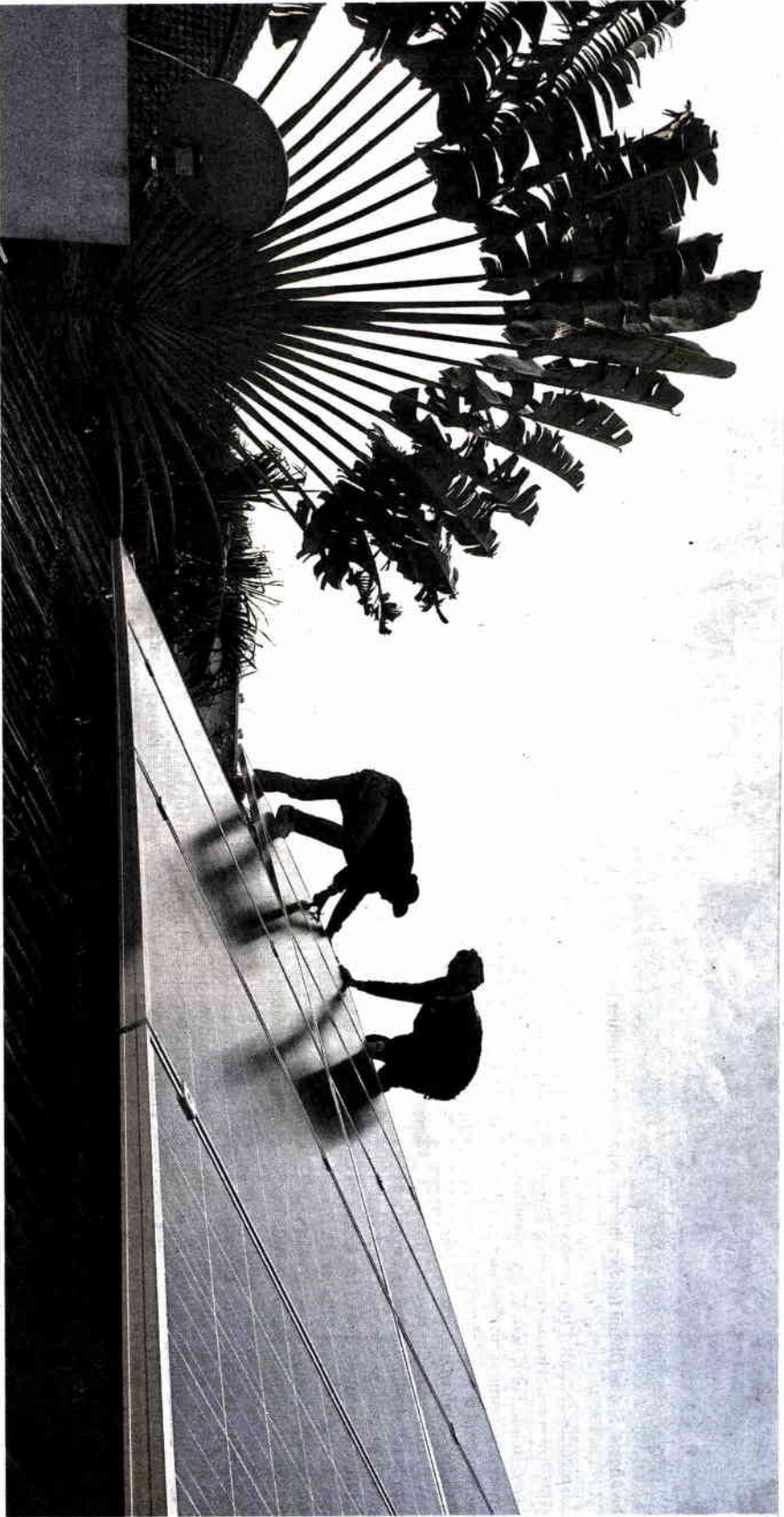
Workers set up rooftop solar power panels. The Energy Ministry recently announced a plan to stop buying more renewable power over the next five years. WEEFABOON WISARTSAKUL
