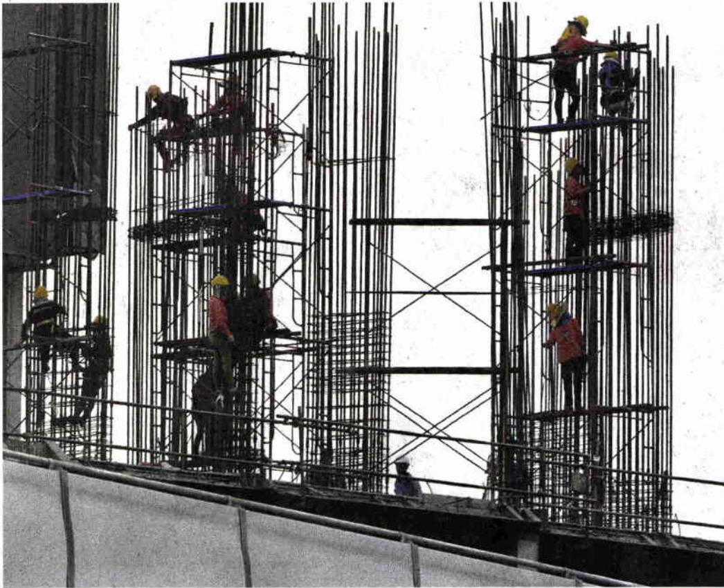
Workers build supports for a condominium in Bangkok. Large structures will be subject to the new energy code when it takes effect this year. PANUMAS SANGUANWONG
