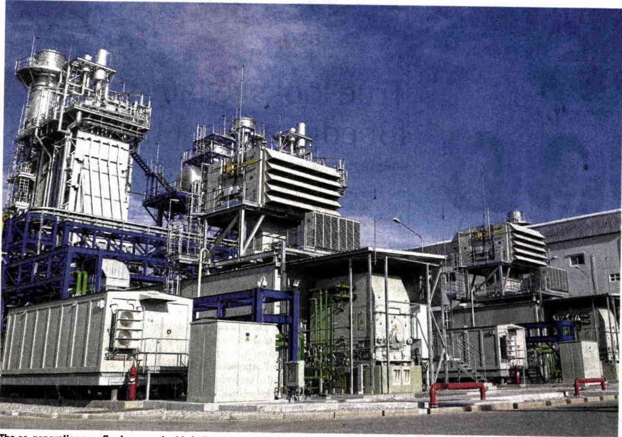
The co-generation gas-fired power plant is in Banpong district, Ratchaburi province.
